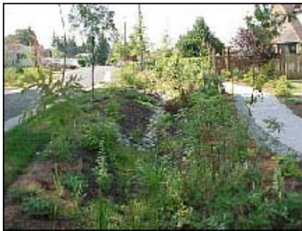
Model Biofiltration swale on Seattle's Street Edge Alternative Project
